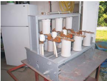
Recondition PDP/SMC style load break switch
